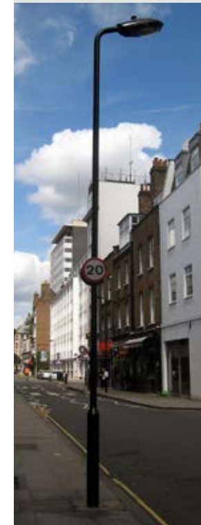
Figure 285: Example of a stepped tubular column
