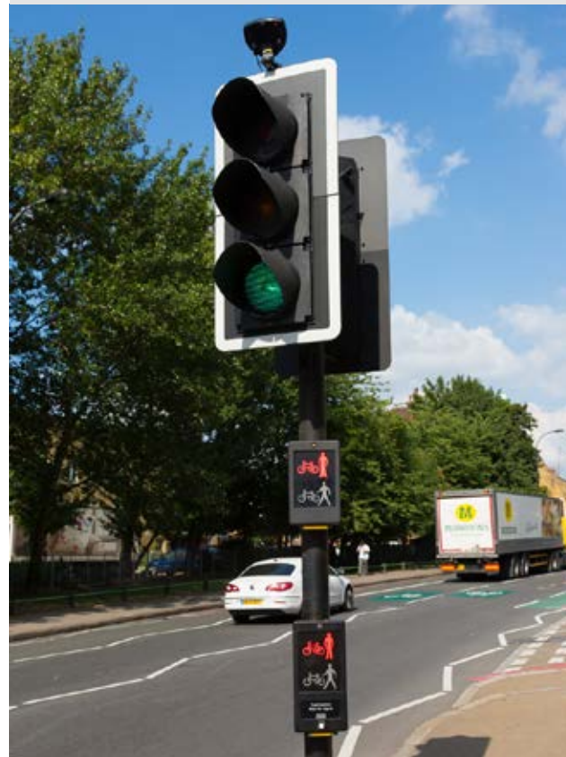
Figure 158: Traffic signal for toucan crossing
