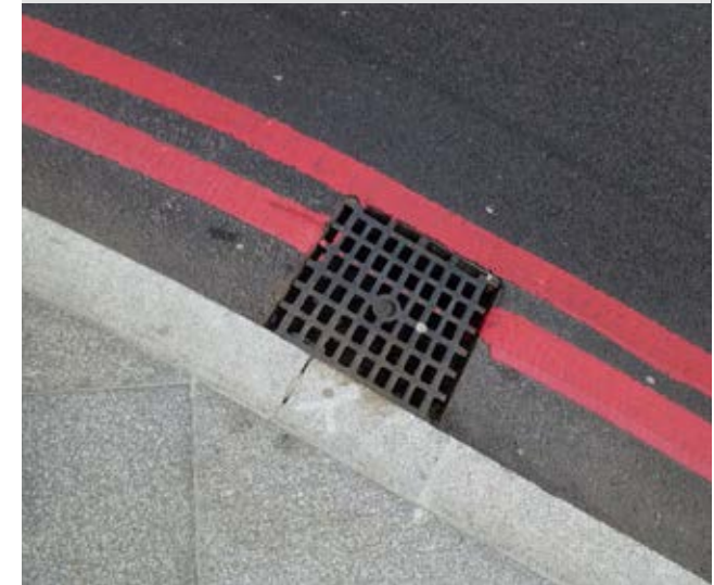
Figure 275: Cycle friendly grate on TLRN
