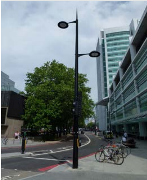
Figure 282: Highway lighting column illuminating footway and carriageway
