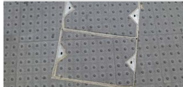
Figure 86: Tactile paving inset into an inspection cover with blisters orientated consistently
