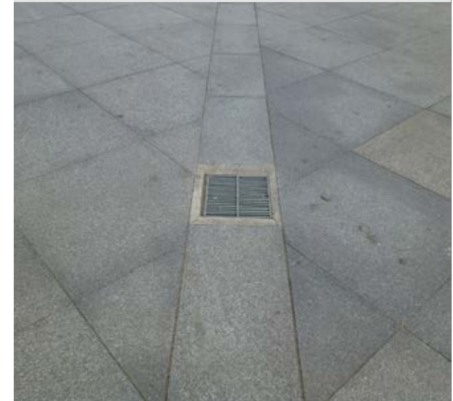
Figure 276: Channel and pedestrian friendly gully
