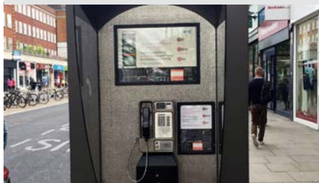
Figure 238: An example of an ST6 telephone box
