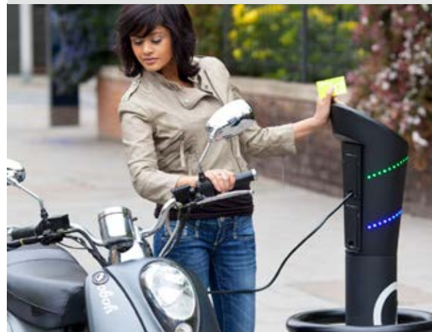
Figure 188: Electric vehicle charging point
