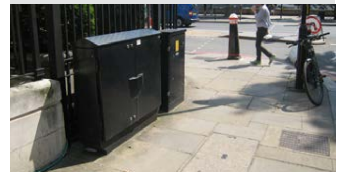
Figure 258: Utility boxes placed at the back of the footway
